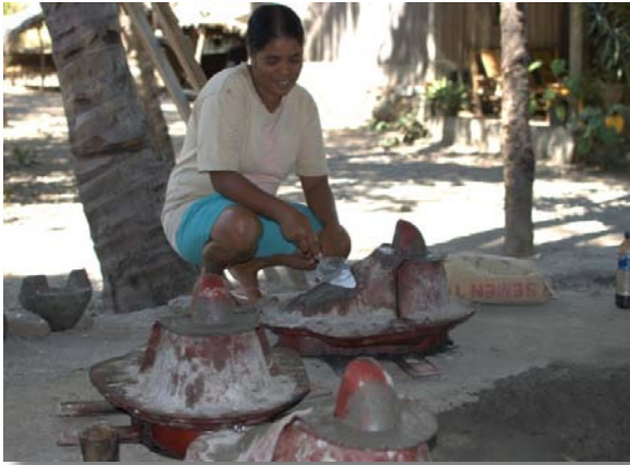
Figure 8: Constructing concrete pans that are used with pour flush latrines in Timor-Leste
