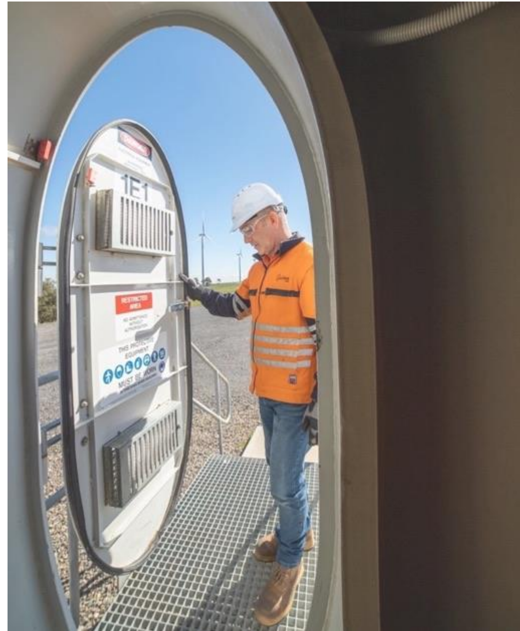
Photograph courtesy of ACCIONA Energy
