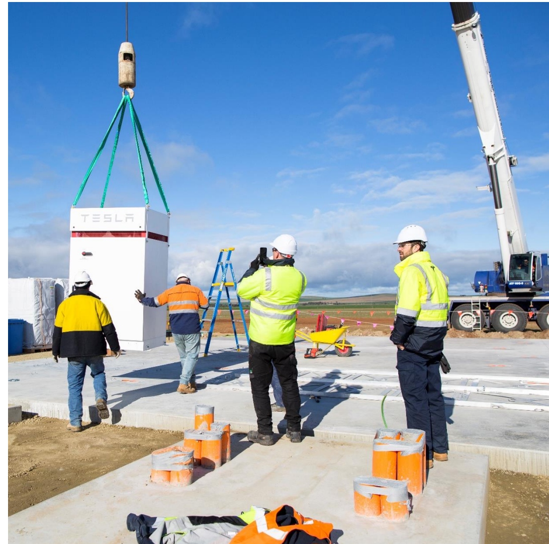
Photograph courtesy of Neoen
