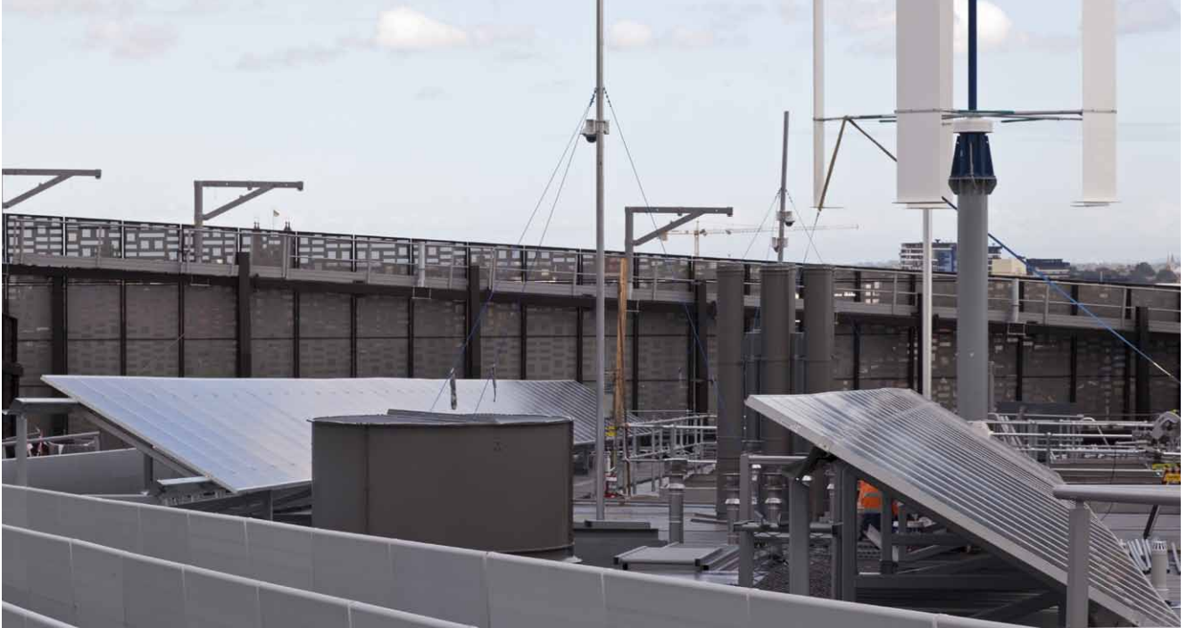
The FEIT Building integrates sustainable features that will not only power the building but be used for teaching and research.
